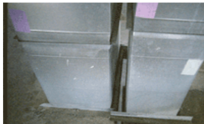
Primary air duct on left and smoke control duct on right.
